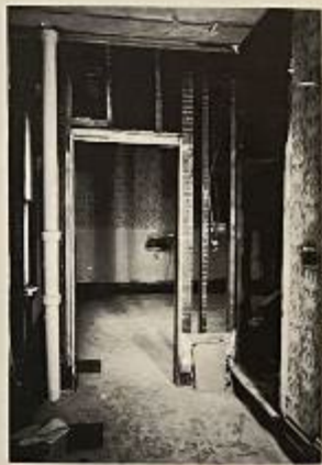
A 'before' picture shows the unattractive view from the bathroom dominating the front hall.
