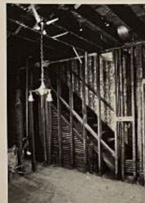
An 'under-construction' picture shows the enclosed stairway being opened up into the living room.
